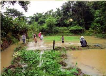
Ditching: here the workforce clear ditches and raise banks in the pouring rain.
